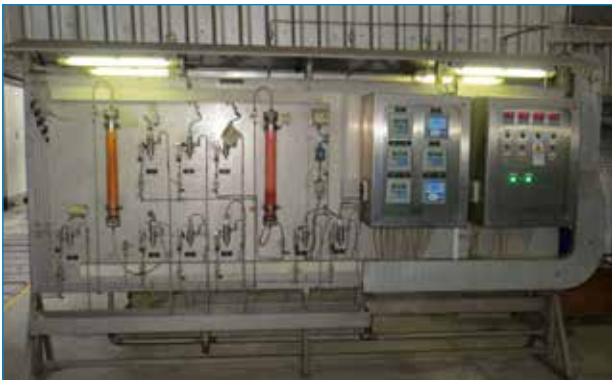
Rack with unprotected wet sensors
