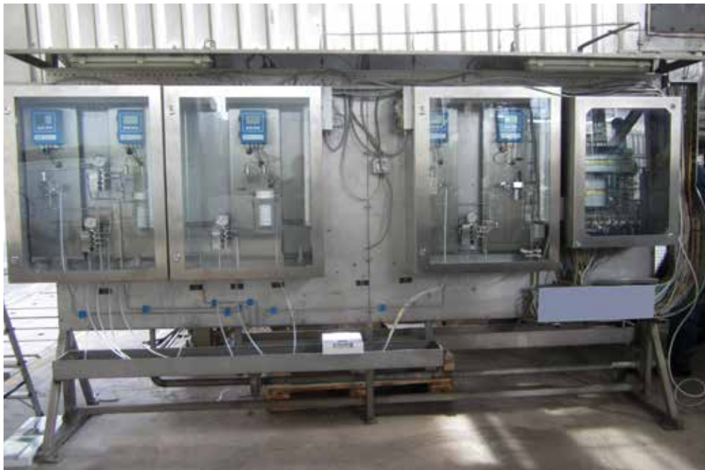
SWAN monitors in protective cabinets
