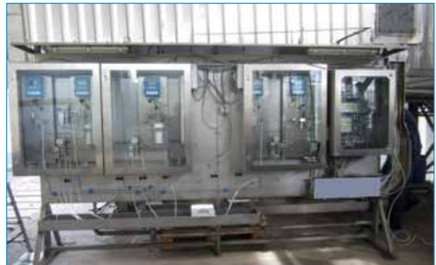
SWAN monitors in protective cabinets
